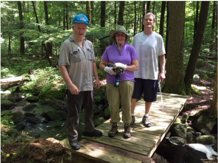
Trails Committee members Charlie Tatham, Anne Melvin, and Doug Winter finishing the bridge
